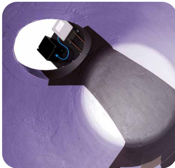
Applied DOPA® technology in an underground tank.
