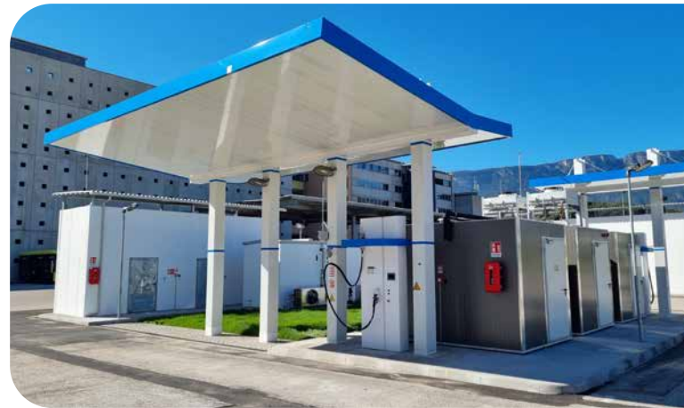
Hydrogen refuelling station developed in Bolzano (Italy).
